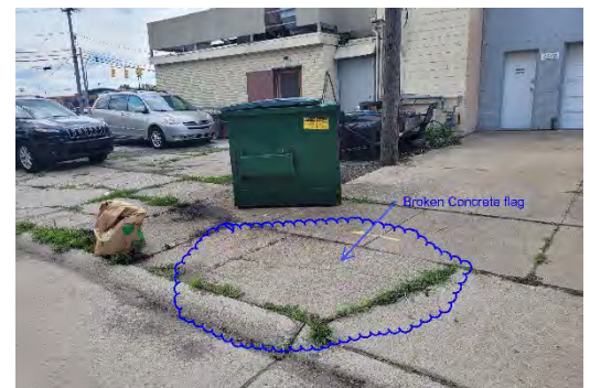
Figure 5: Concrete flag in back of building.
